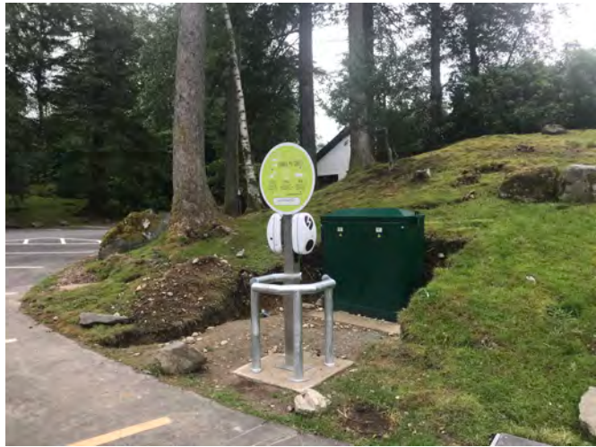
1 New charging point at Langdale in Lake District
